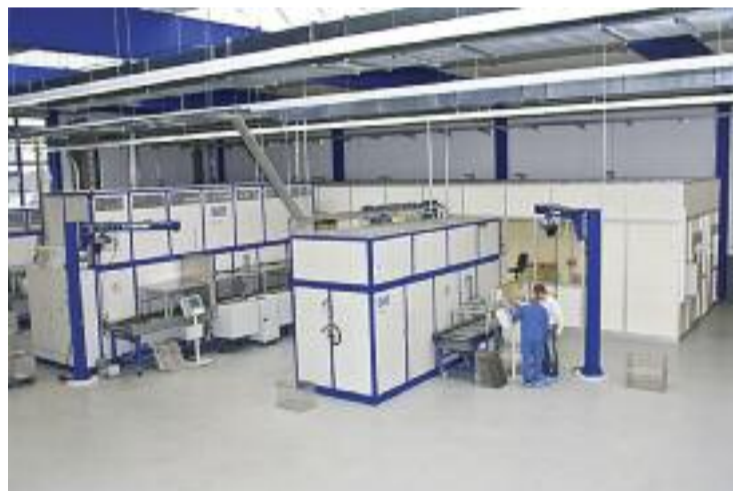
Cleaning plants connected to a cleanroom
